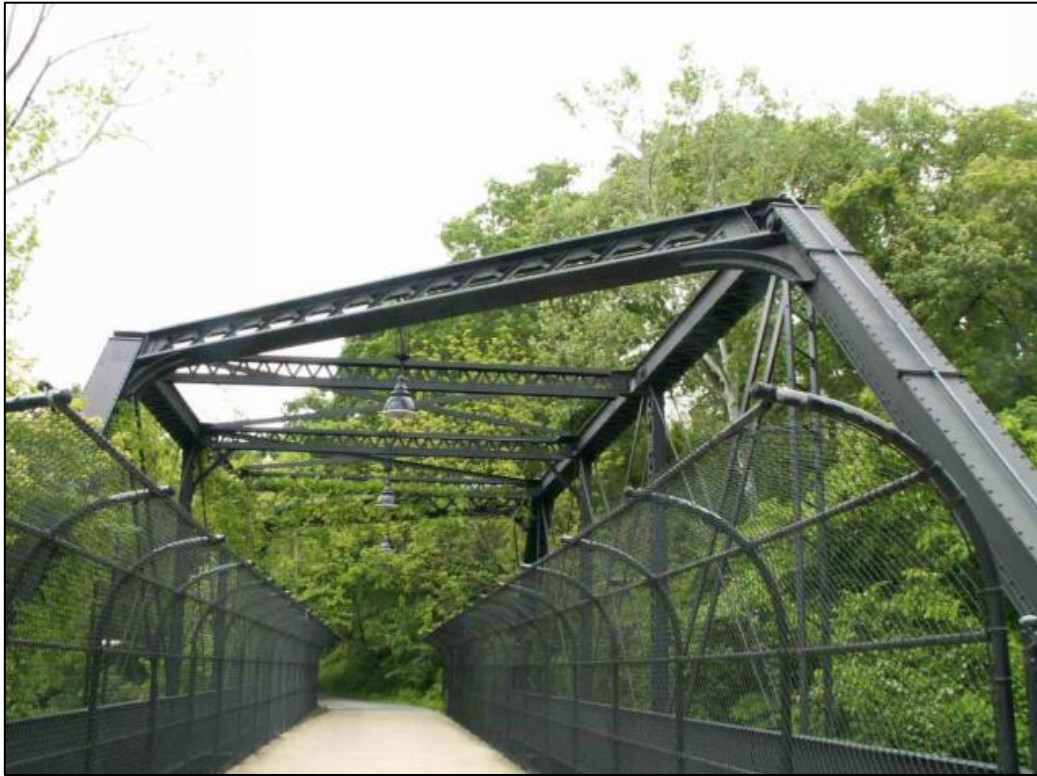
Photo 8 – 10 Years after Application of Termarust
