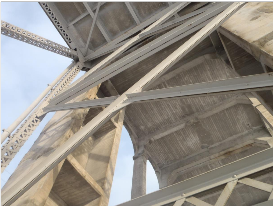
Photo 7 – 10 Years after Application of Termarust
