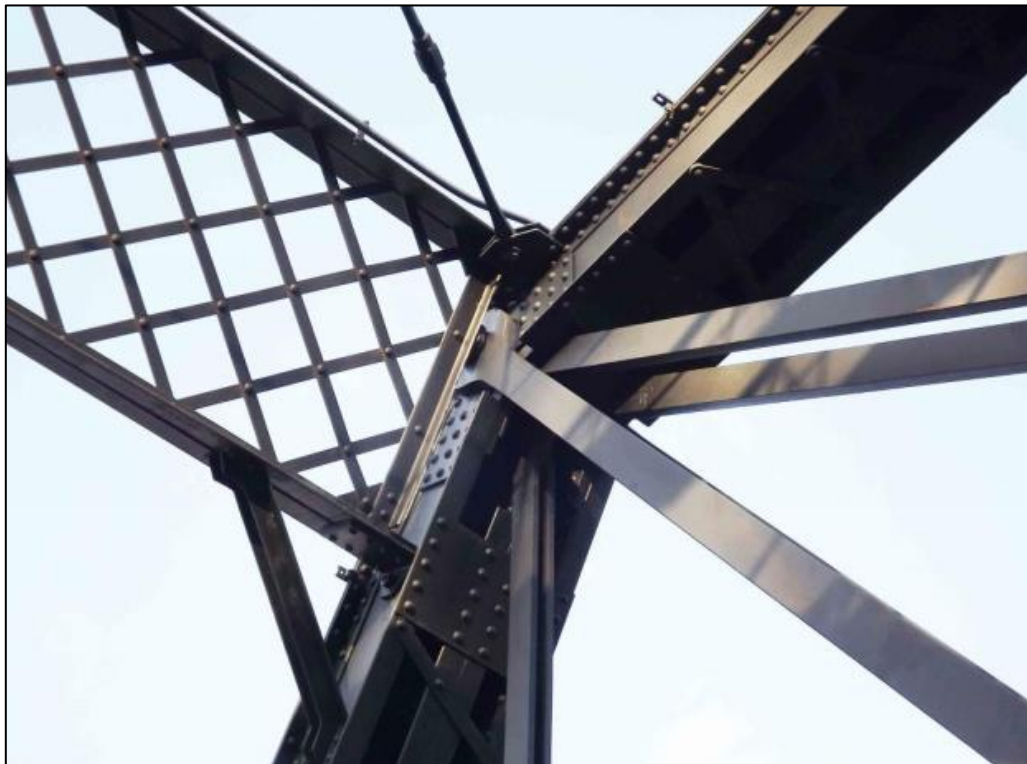
Photo 9 – 15 Years after Application of Termarust
