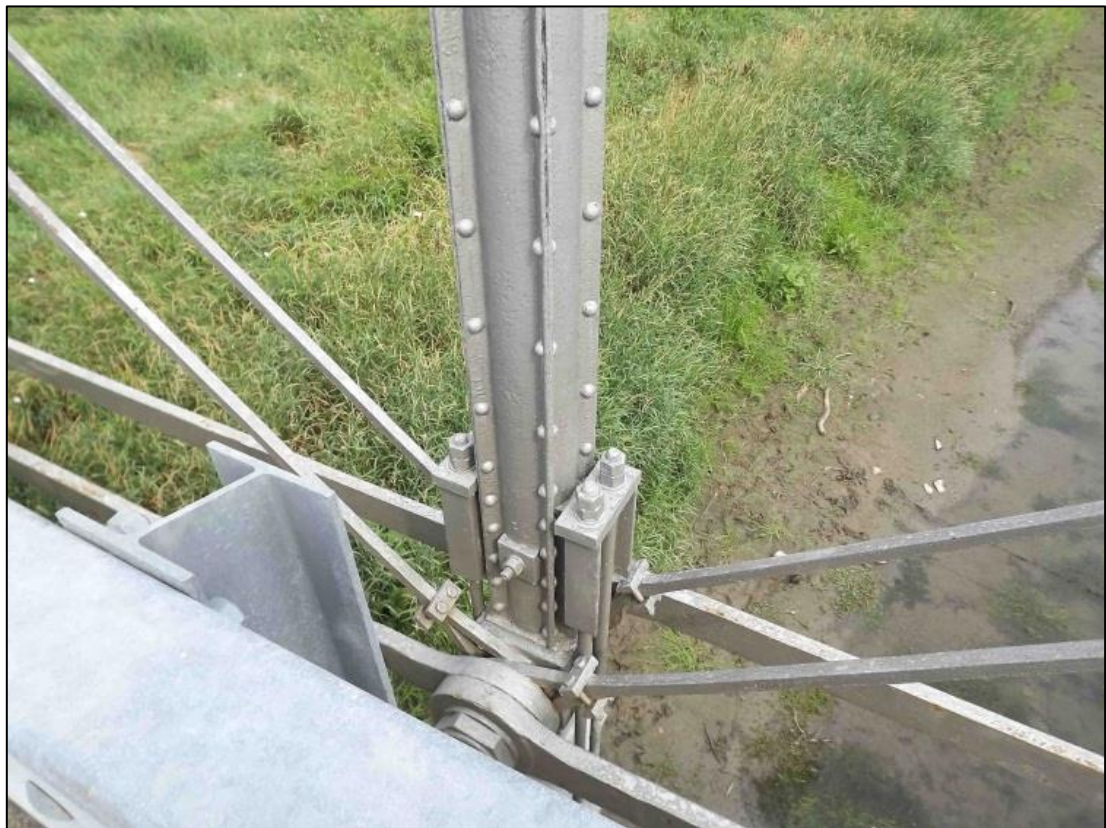
Photo 5 – 8 Years after Application of Termarust
