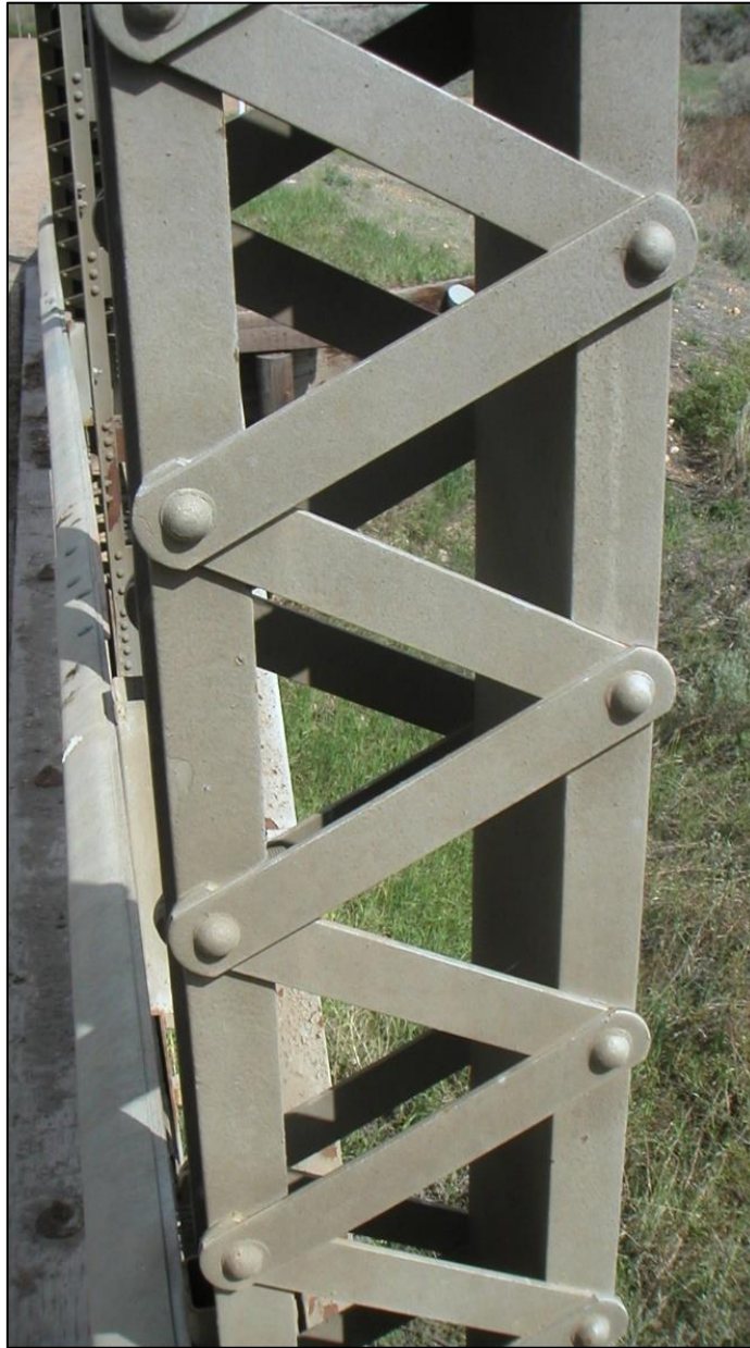
Photo 10 – 22 Years after Application of Termarust
